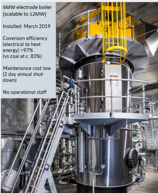
Figure 77. SML Dunsandel: NZ's first large-scale electrode boiler
